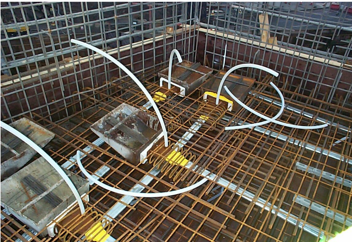
Figure 9. Post-tensioned floor slab system prior to casting concrete with flat tendons (white) and live end anchorages in pans set in from the slab edge. Also visible are white grout tubes and yellow seals joining the ducts to the anchorages. The unstressed strand tails can be seen projecting from each duct within the pans.
