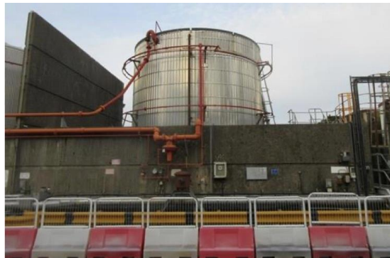
Photograph 6 - One of the Four Gas Turbine Fuel Tanks
