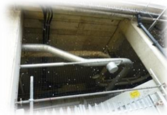
Netting to prevent bird access
