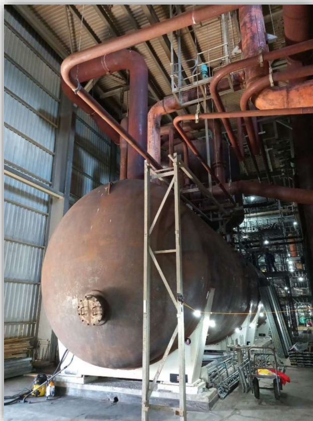
Photograph 9 De-aerator tank and associated pipework post removal of insulation containing asbestos and Haki staircase removal.
