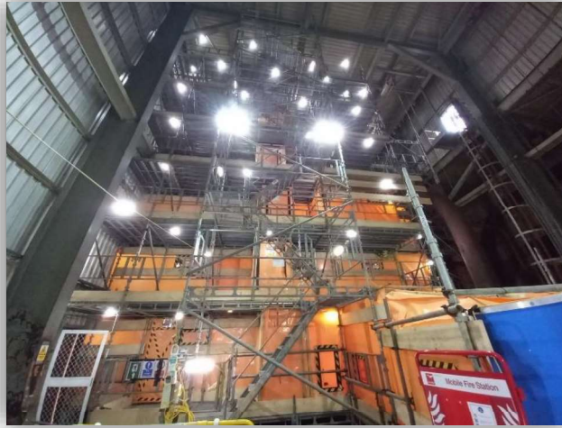
Photograph 7 Asbestos tented area enclosure with airlock and negative pressure air system & decontamination unit
