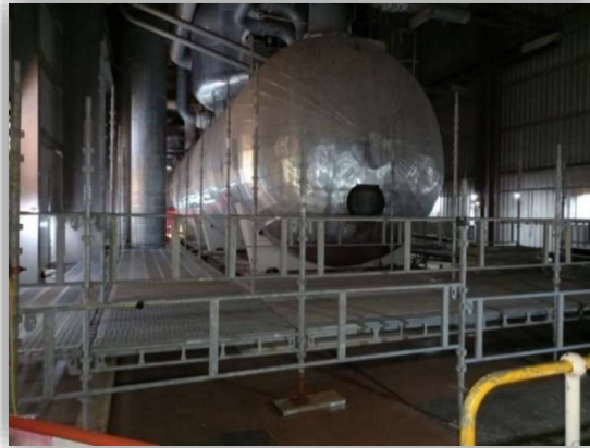
Photograph 5 De-aerator tank with associated pipework with insulation containing asbestos.
