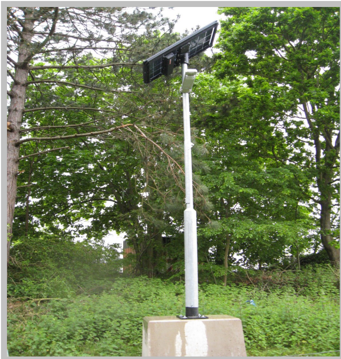
Figure 3: Solar Lighting Towers
